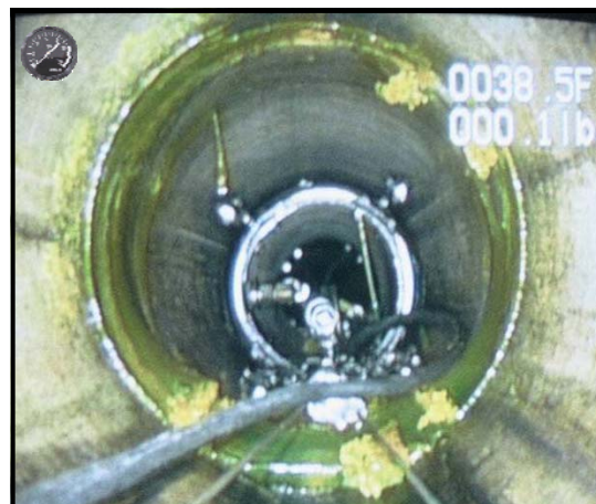
Minimal residual grout ring remaining
