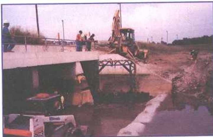
The packer awaits launch in the box culvert which was filling with sand from failed joints.
