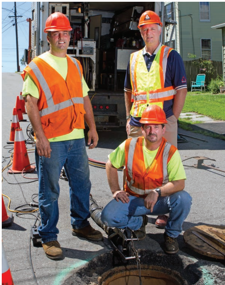
The New England Pipe Cleaning crew includes (from left) technician Jason Mahler, general manager Michael Poplawski and crew leader Charlie Roberts. They are shown with Logiball lateral sealing equipment.
