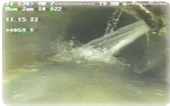
Infiltration at lateral connection
