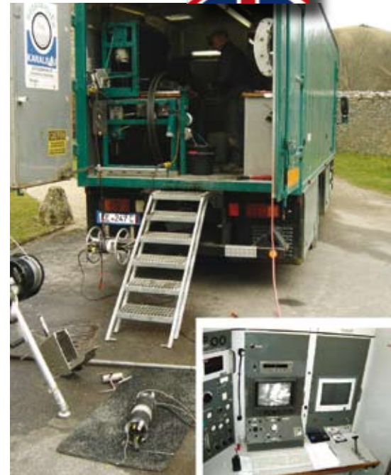
The Acrylate Injection joint sealing truck with the sealing packer being prepared behind it and (inset top) the control cabin set up within it
