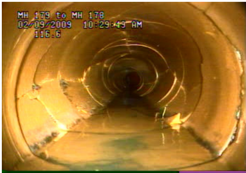
Figure 4 – Broken Pipe (Courtesy of Township of Falls Authority)
