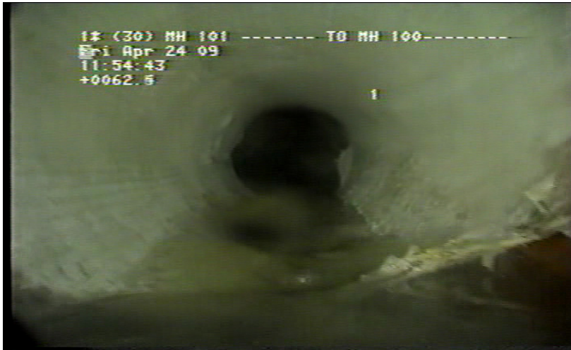
Figure 5 – CIPP Liner Point Repair, 3-foot length (Courtesy of Township of Falls Authority)
