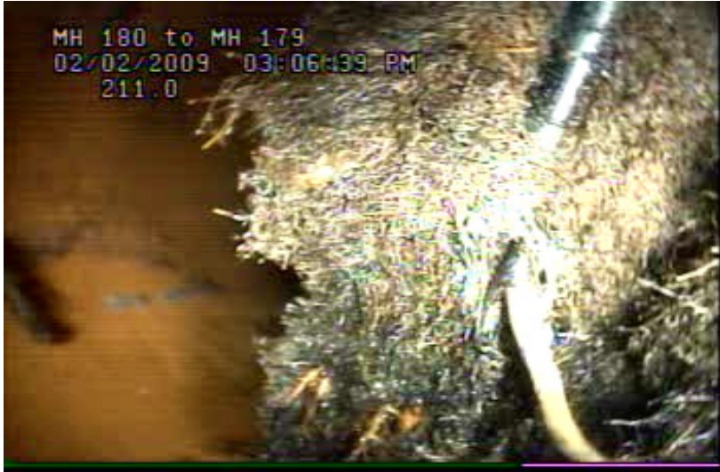
Figure 1 Root Ball in Pipe Segment MH 180 – MH 298 (Courtesy of the Township of Falls Authority)
