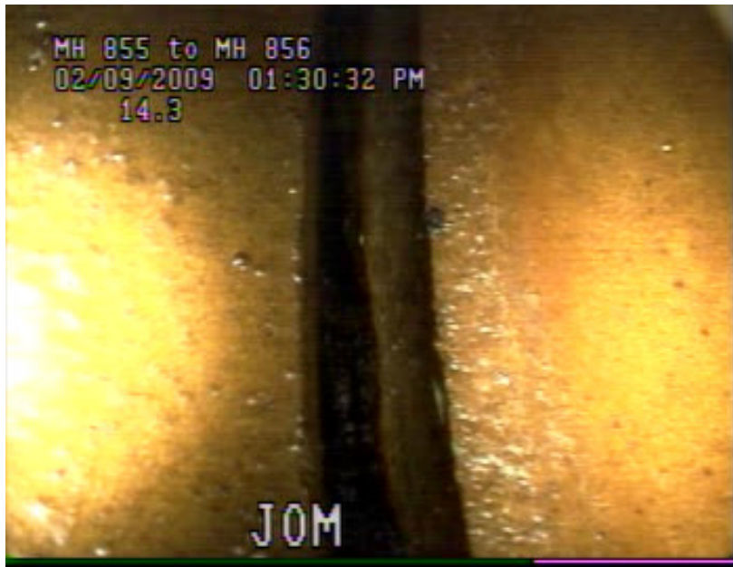
Figure 3 – Open Joint / Joint Offset (Courtesy of Township of Falls Authority)
