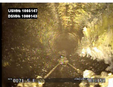
Barrel of the siphon, horizontal run, note heavy grease present
