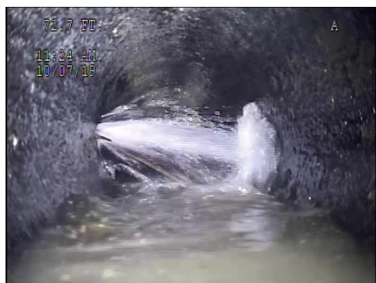
Once the siphon was cleaned the leak could be readily seen coming in from the river above.
