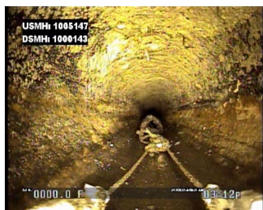
Photo of siphon just outside of The start of the siphon structure Here the camera is traveling Down the incline of the siphon
