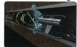
Leaking joint in mainline sewer
