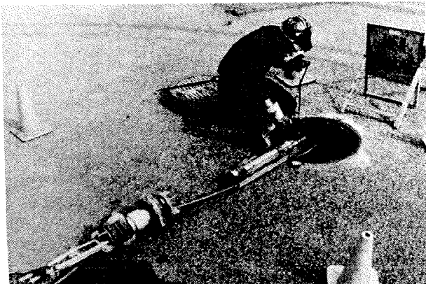
Dropped through manholes into successive sewer line sections, rehabilitation was done by a grout injector packer, left, guided by a closed-circuit TV inspection camera, right.
