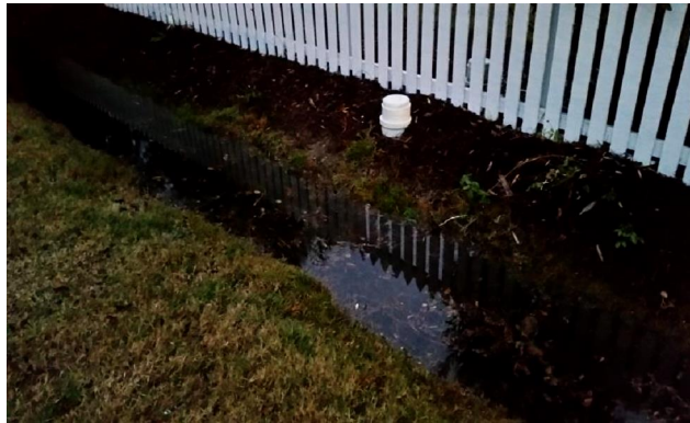
Figure 6 – Lateral Under Water-filled Storm water Swale
